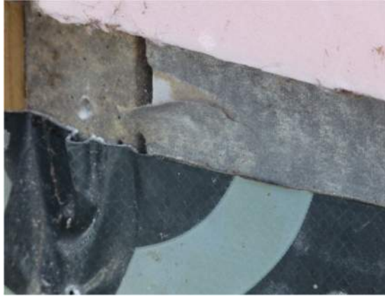
Paper-faced sheathing is showing some signs of damage where exposed to the water plane.
