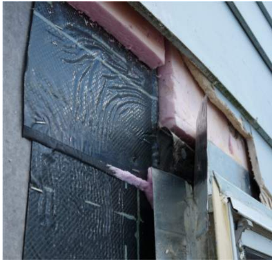
Window blocking has been wrapped with a vapor barrier product, mechanically fastened to the sheathing behind the insulation.
