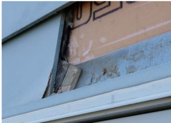
Gypsum board used as a spacer at the window head to hold siding off head flashing.
