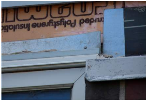
Flashing joints at the window head and the top of masonry transition do not overlap and are not sealed.
