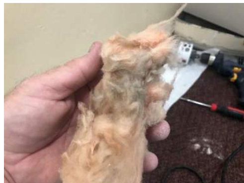
Batt shows no indication of water infiltration into wall cavity.
