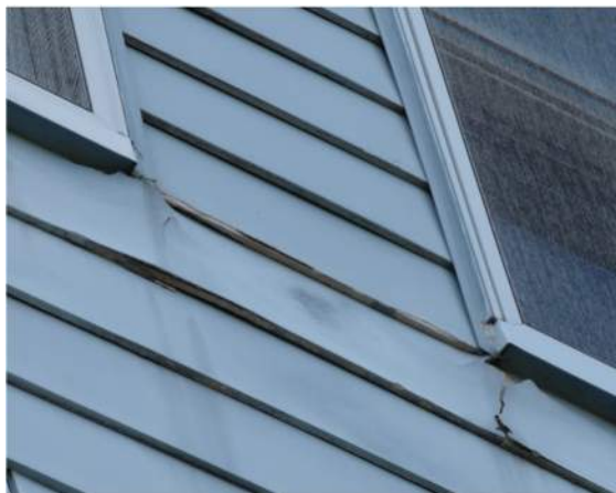
Damage to the siding at the outside sill corners of the windows indicated that water trapped in the j-channel at the head of the window eventually travels down the jambs, seeping into the siding.
